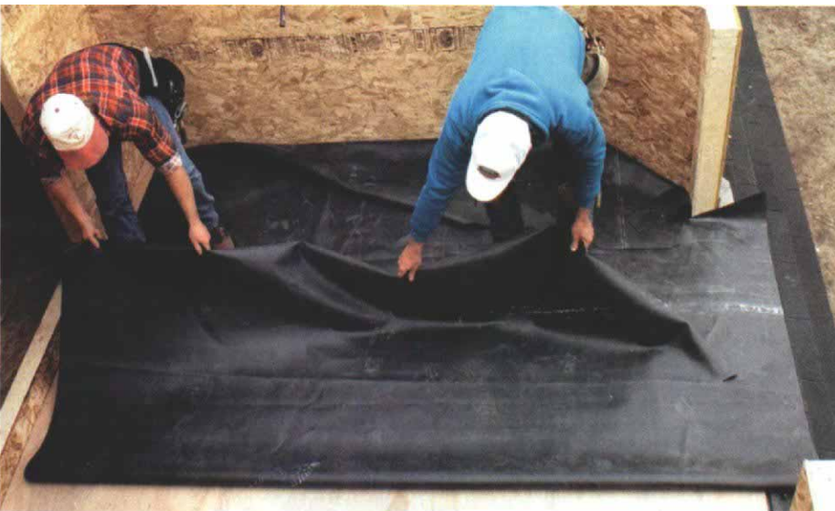
Unrolling the membrane for a dry fit. After the substrate has been prepared properly, the sheet of EPDM is laid out in the area to be covered for a dry fit.
