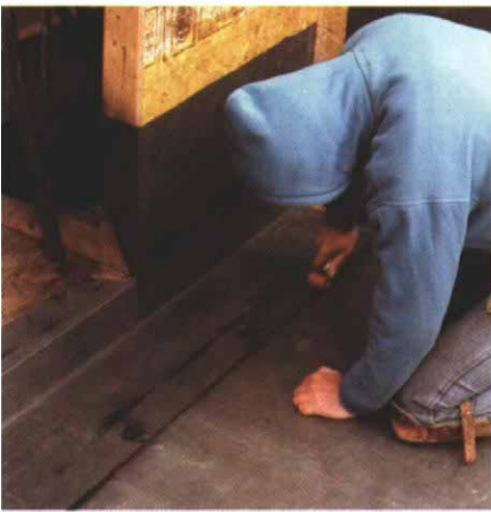
Rubber-to-rubber glue for the overlap. A special contact cement glues down the overlapping area of the splice. The small dabs on the face helped to stick the membrane up out of the way while the glue was drying.
